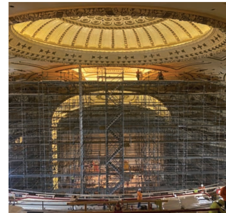
MARCH 2024 Scaffolding fills much of the auditorium as cleaning and painting begins.
