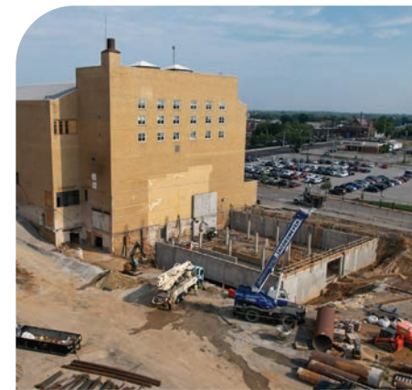
AUGUST 2023 Crews pour and finish the basement floor of the new backstage wing.
