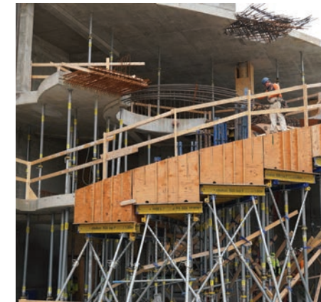
JUNE 2024 Form work for the spiral staircase in the new front of house expansion begins.
