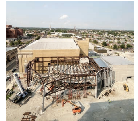
JULY 2024 Crews begin building the steel shell that will envelop the expansion.
